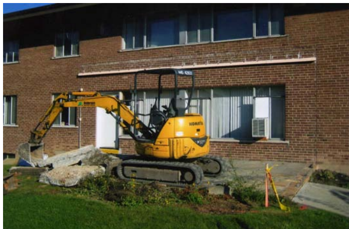
Renovation work continues at The Lighthouse, with completion anticipated in January. A bequest by the late Bernard Leising provided $100,000 to enhance the parish Outreach Ministry.
