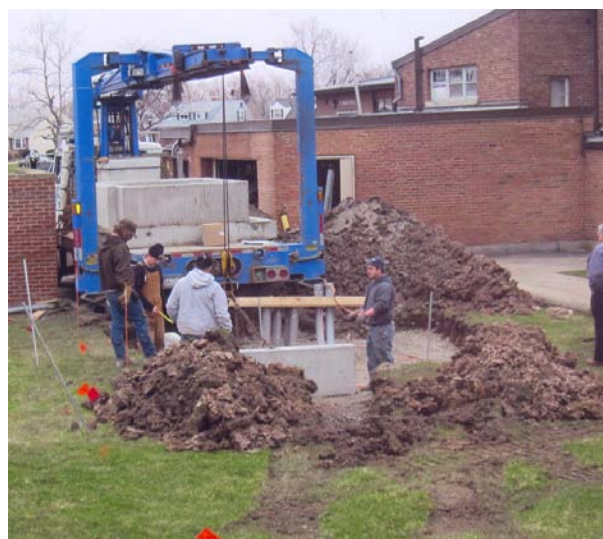
Workers install a concrete base, conduit, and cables for a new electrical transformer adjacent to the gymnasium, which will ensure the parish has adequate electrical capacity for future needs.
